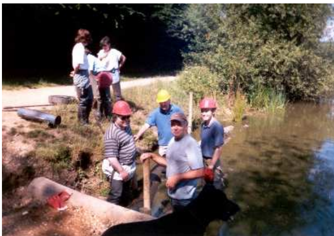
Above left, left & below right – joint task with WMCV at Dinton Below left – Finished revetment at Dinton 14/7.
