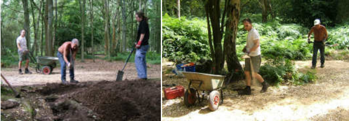
Above left – Phil & Aimee look on as Richard mattocks out the second drainage ditch.
