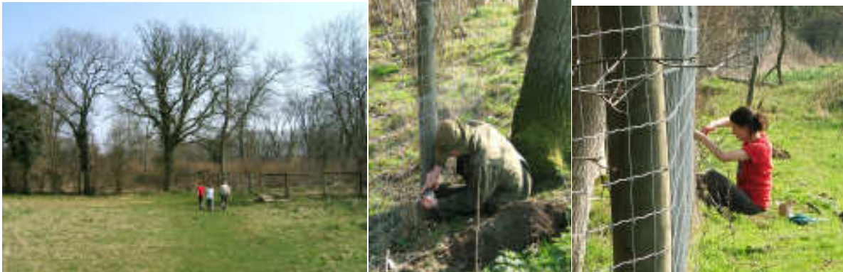
Above left – Fran took us on a short guided walk around the site. Above middle – Phil repairing a hole in the fence. Above right – Fran doing the same.
