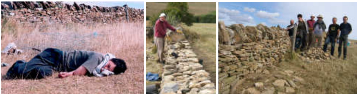
Above left – enjoying a well earned rest! Above middle – Maurice putting on a coping stone. Above right – the team in front of the finished wall.
